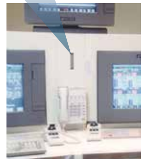
SIS Indicator in control room.
